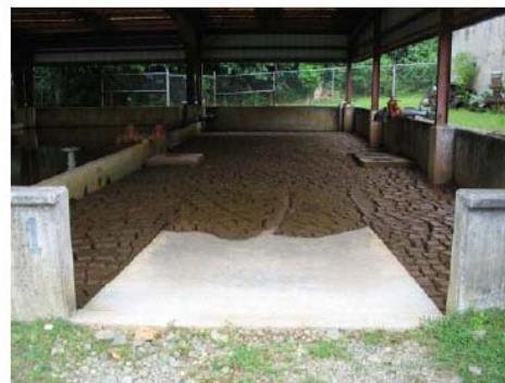
Sludge drying bed
