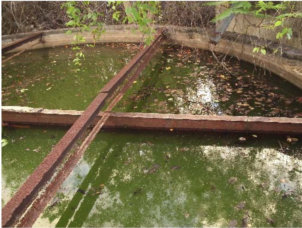
Fig. 2.1 Ferrocement rainwater collection tank in Banaba. The absence of a roof means that water is exposed to sunlight and organic debris such as leaves. Algal blooms result and the water is unused (Photo Moiuva, WEU, MPWU).
