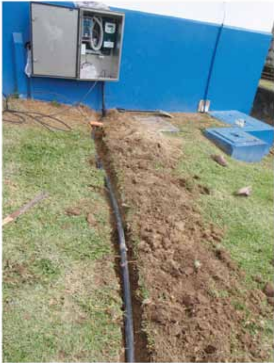
Tagabe Stream, Efate, installing pipeline and instrument at main water supply pumping station
