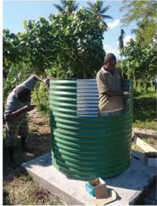
Assembling security housing for instrumentation, La Colle River
