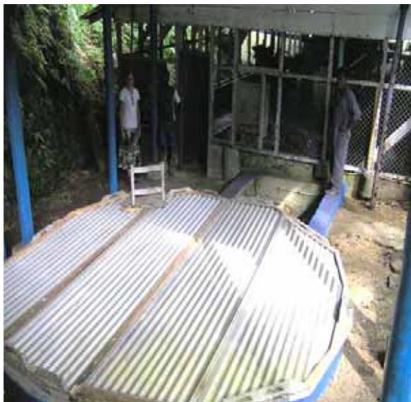
Luganville water supply intake well
