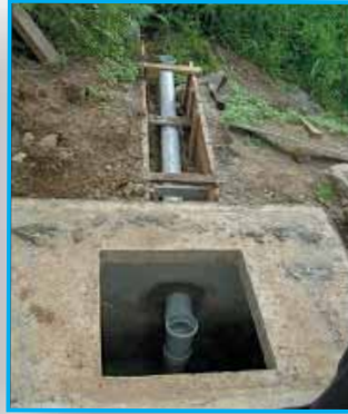
Septic tank and soakage trench with viewing portal (3)
